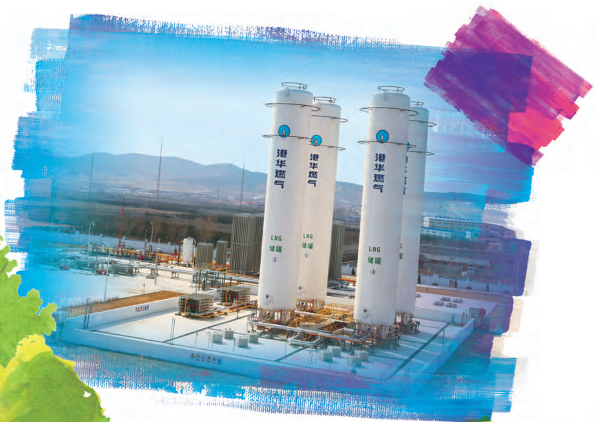
Liquefied natural gas tanks located in Dalian Lvshun Hong Kong and China Gas Company Limited
