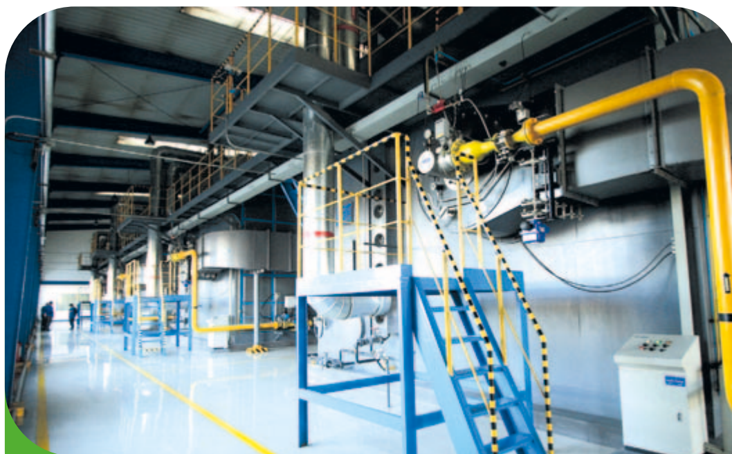
Gas equipment of China First Heavy Industries (Group) Co. Ltd, a customer of Qiqihar Hong Kong and China Gas Company Limited.
