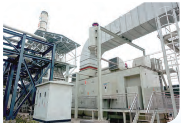
Snow Brewery in Xindu district, Chengdu City of Sichuan Province has installed a distributed energy system that makes use of natural gas to generate electricity and residual heat for cooling and steam production. This marked a new era for energy efficiency and productivity.
